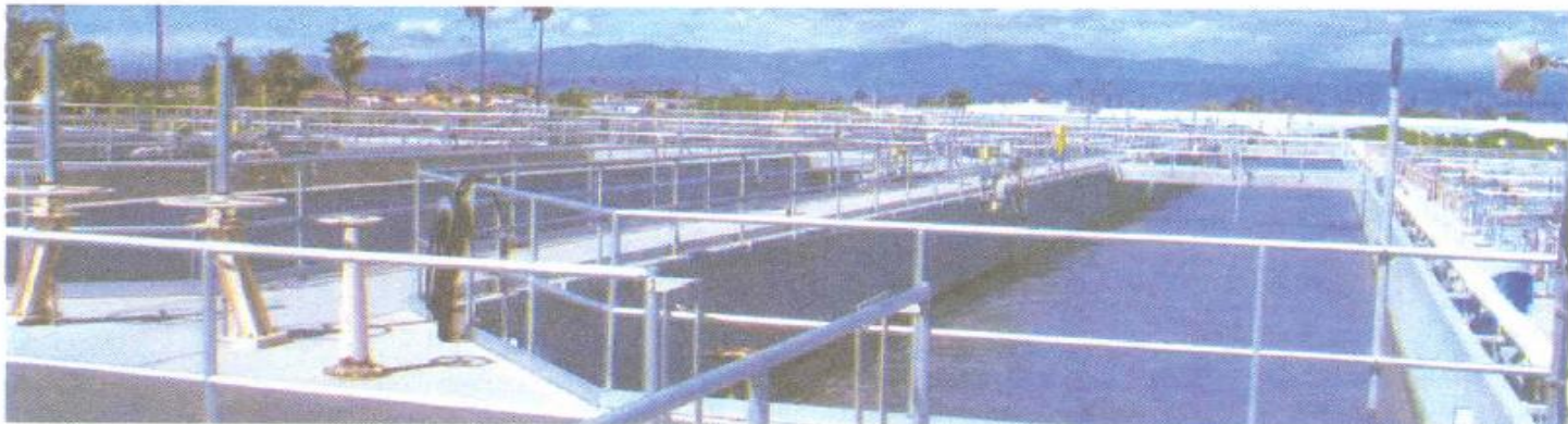
Loji pengolahan air sisa. Wastewater treatment plant.
